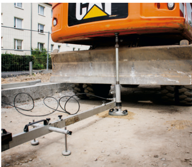
Figure 19 Plate bearing test according to DIN 18134 with a 300 mm diameter load plate
